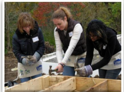
SWE members volunteer their construction and teamwork skills for Habitat for Humanity's Women's Build
